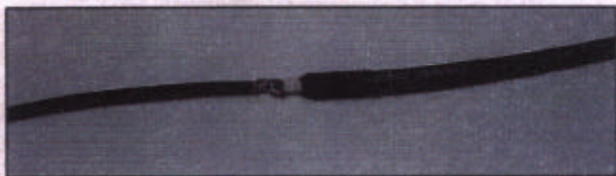
Photo B— Connection of inner end of coax section (closer to center). Note that only the center conductor is connected to the wire.
